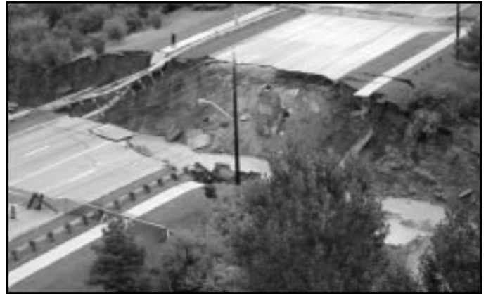
Finch Avenue blow-out during the August 19, 2005 storm that rolled through Toronto wreaking havoc. Photo Courtesy of RiverSides.
